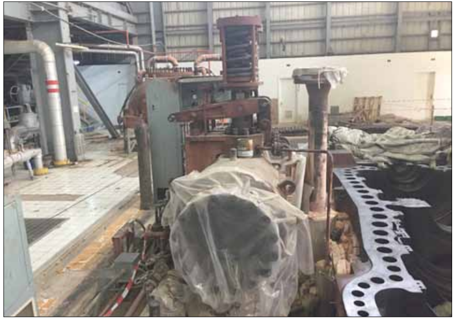
At the Aleppo power station, all five turbines were destroyed bei ISIL. Now they are repaired by hand. Turbine 5 was put back into operation in summer 2022. (picture Karin Leukefeld)
