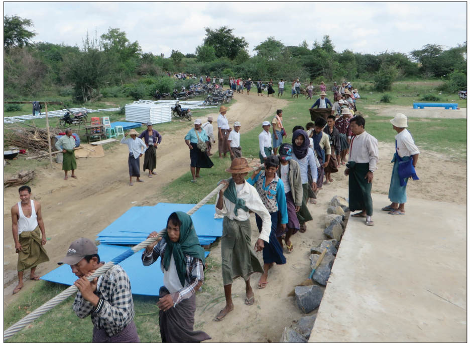
The ropes are among the most important components for building a bridge. Everyone helps with the transport, here in Ywar Wai, Mandalay in Myanmar. (picture Toni Rüttimann)
