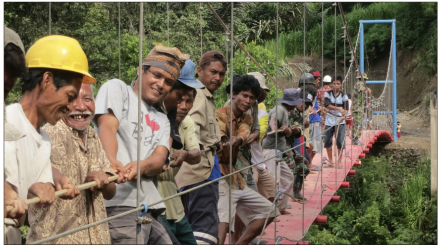
Pulling together: Trust in cooperation and engineering expertise make this bridge possible. (Picture screenshot; https://vulcanostatale.it/2016/01/serial-bridge-builder-a-conversation-with-toni-ruttiman/ )
